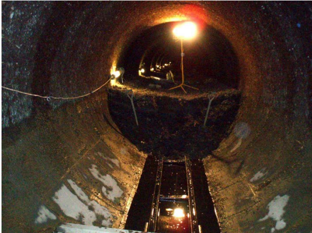
Figure 1. Blockage of a raw water pipe in southern England showing an accumulation of zebra mussels that have half-blocked the pipe.
